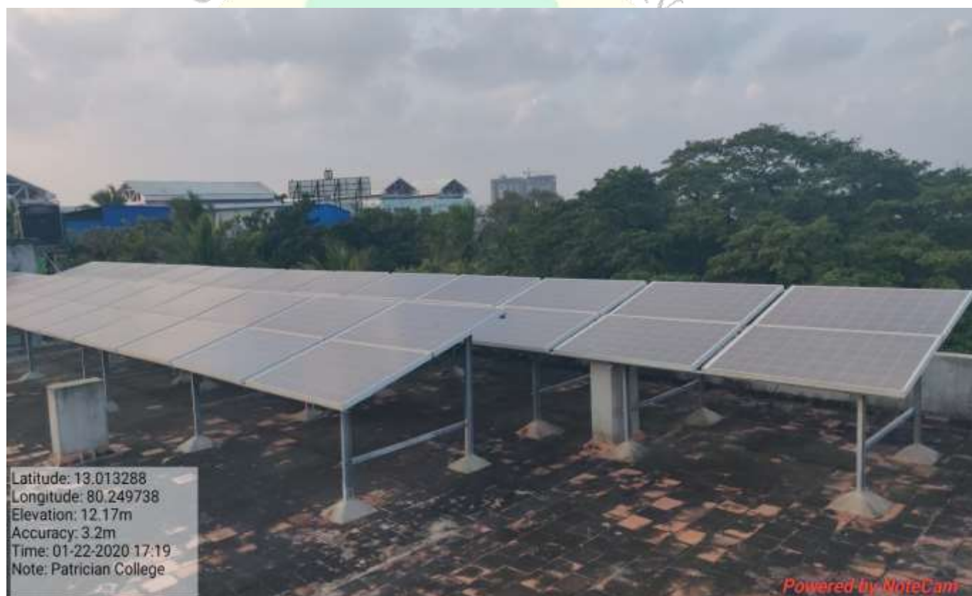
Solar Panels – B Block
