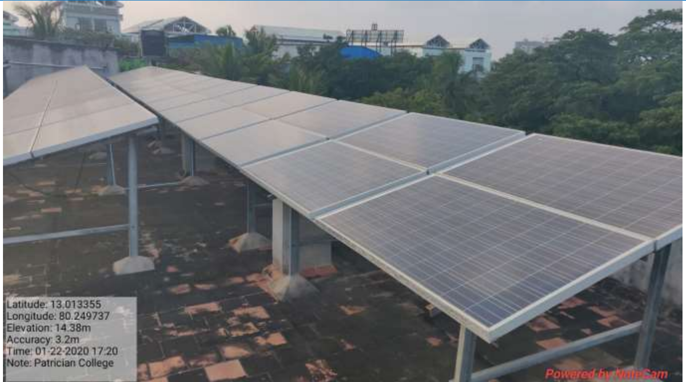
Solar Panels – B Block
